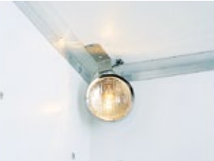
⑨室内作業灯
